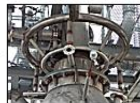
Partial oxidation of separated pyrolysis gases and vapors, for primary tars conversion and abatement (vortex partial combustion reactor)
